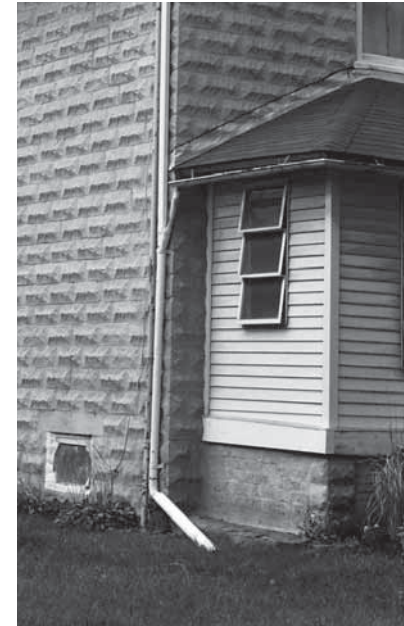
Avoid enclosing porch openings with siding materials. In this example the porch has been completely enclosed to make an extra room.
