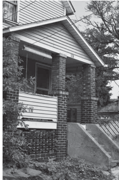
Maintain the house's original wood siding wherever possible. Here the clapboard balustrade has been covered in vinyl siding.
